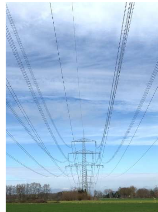
Transmission power line (ref: DLR)
