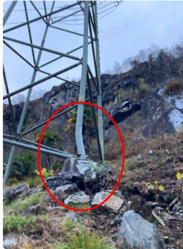
Boulder impact at pylon 1900x006
