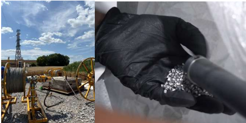
Rte Installation of a Recycled Aluminium Alloy Conductor on RTE's Grid, 27th May 2026
