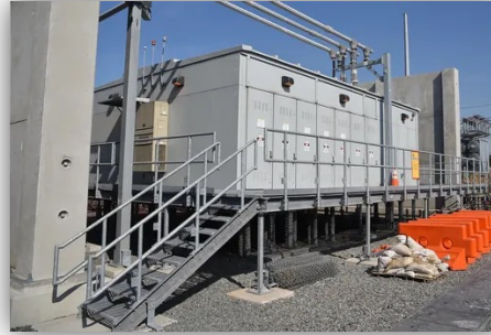
PSEG Substation Newark, USA
